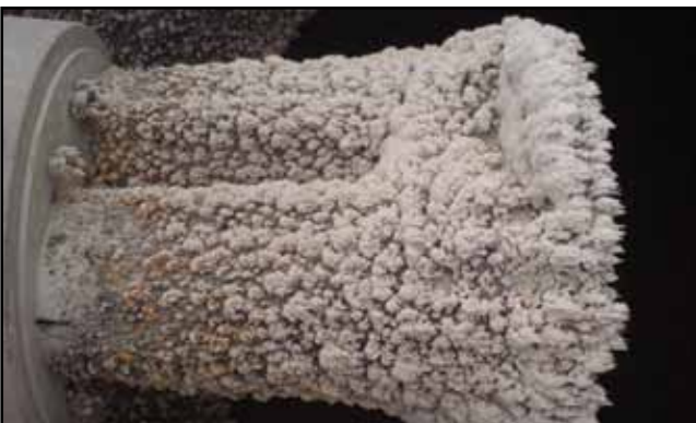
Outer unit is coated with build-up from dust.
