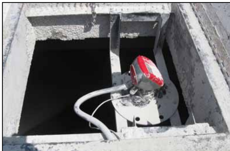
A dusty application in an ethanol plant.
