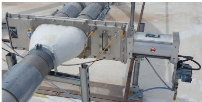
Ceramic backing on a pneumatic diverter inlet
